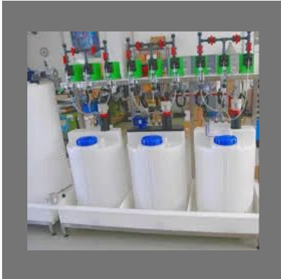
Chemical Dosing System
